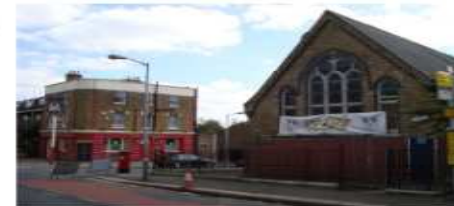
Problems have meant that it can no longer be used without significant remedial work, and it is now standing empty
